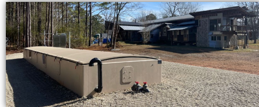
Decentralized system installed in Newbern, AL
